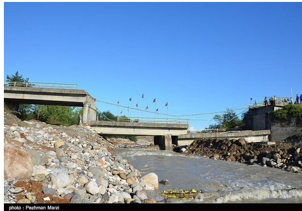
photo - Pezhman Marzi Fig. 2. Damaging and destroying the existing structures in Shiroud River
