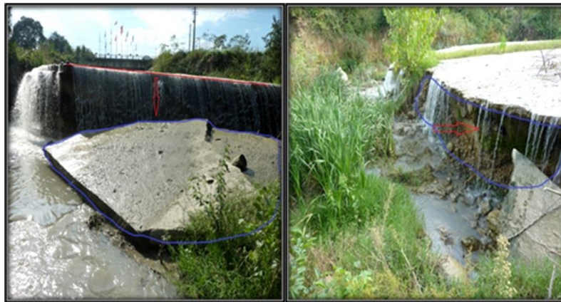
Fig. 8. Destruction of short drops constructed on the river bed to prevent degradation in Lavij River
