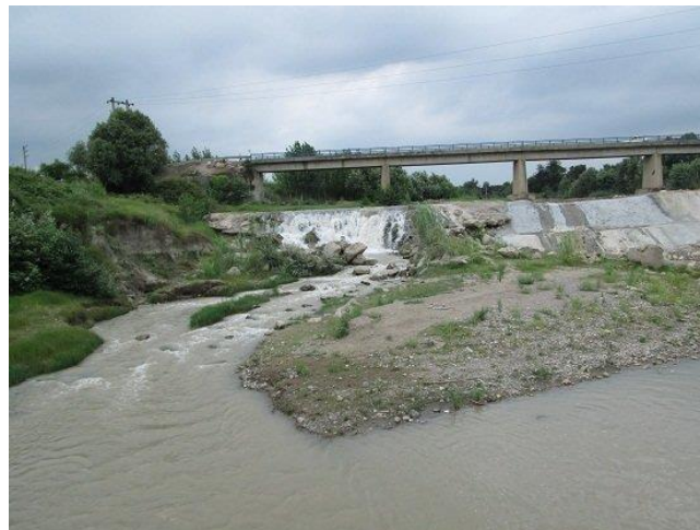
Fig. 3. Increased the slope and caused a breakage in the river bed in Talar River
